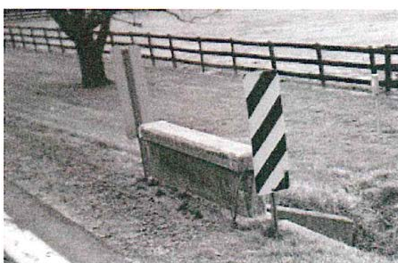
This headwall is a roadside obstacle and should be replaced as soon as possible.
