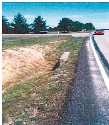
This culvert headwall is a roadside hazard.
