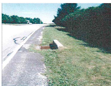
The headwall is sticking up almost a foot in a relatively flat recoverable area. It can snag a vehicle and bring it to an abrupt stop or cause it to overturn.
